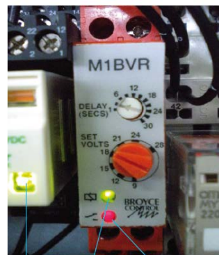
Relay BoSS ON Contact relay BoSS ON Control relay battery ON
